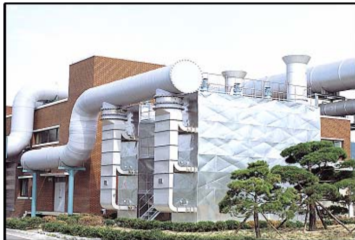
Figure 11. Long view of BIOSAINT biofilter installed at Busan Janglim POTWs
